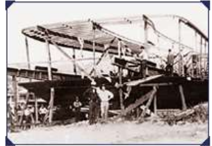
The Idlewild under construction. She has outlived the men who built her
